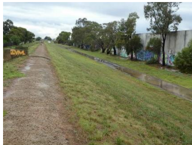
Flooded bike path behind shops on N side of Old Geelong Rd, Hoppers Crossing. Upper (curved) paved section is interrupted with square hatches to access buried pipeline (I reckon), so not good to ride on. VicRoads responsibility.
